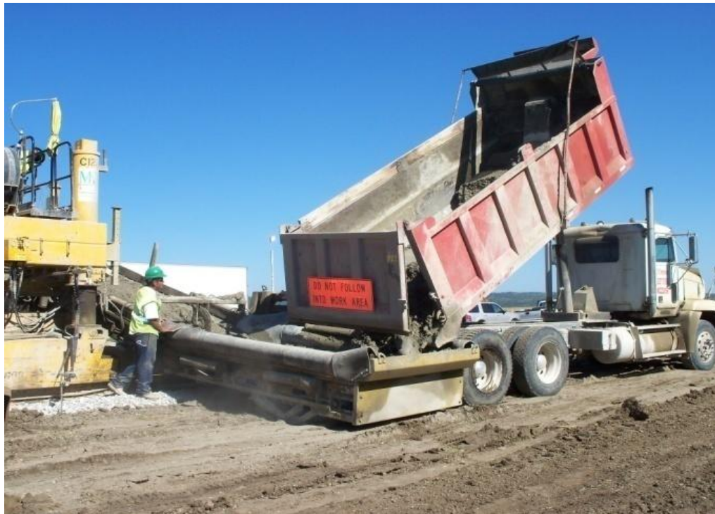
Figure 6 Concrete being dumped into a belt placer and spread by the placer.
